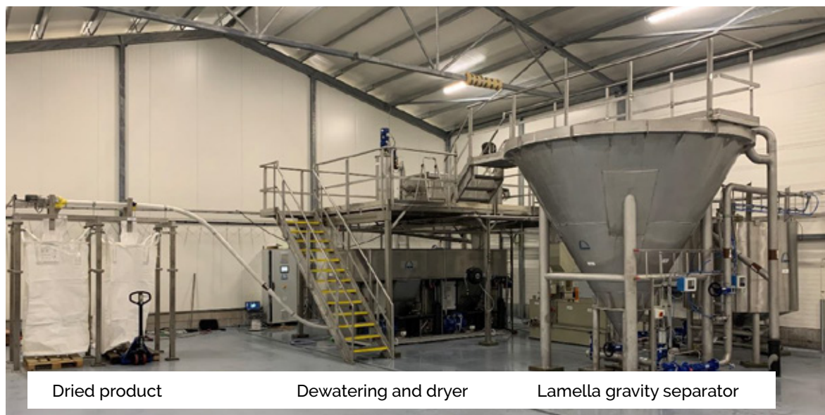
Fig. 5 Osland MAT sludge treatment plant
