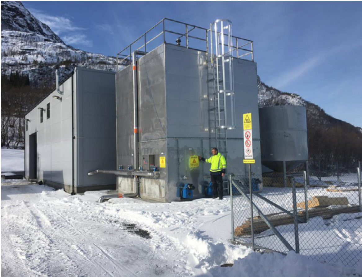
Fig. 10 ABR anaerobic reactor (100 m 3 ) at Forsan
